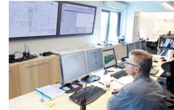
Operators in control room. The facility is designed to run on auto-pilot nights and weekends, so there is a high level of instrumentation and control. ▼
