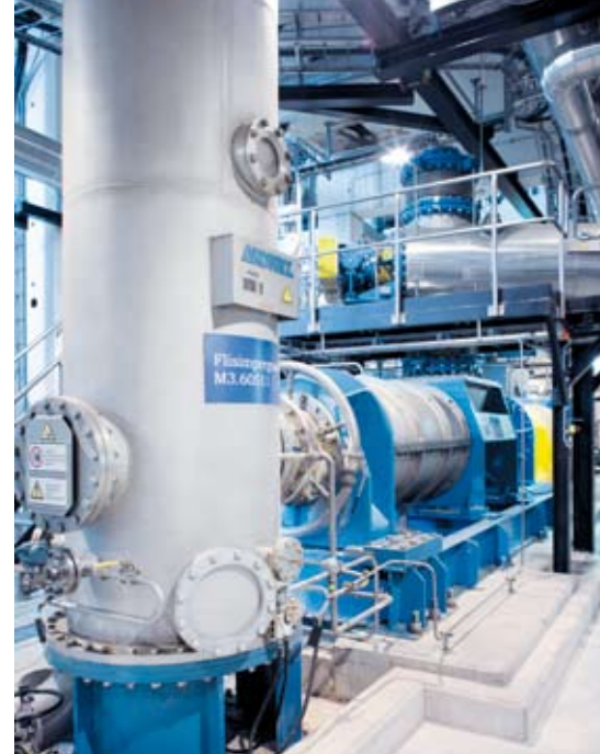
▲ Part of the RT-pretreatment technology at Holmen Paper Braviken mill.
