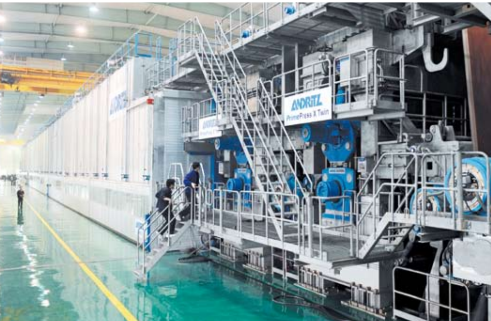
◀ ANDRITZ's machine includes a multi-layer PrimeForm former and a PrimePress X Twin. A PrimeReel is used for winding parent rolls up to 3.6 m maximum diameter.
