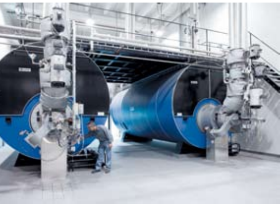
▲ Two gas boilers at the plant can also utilize the product gas from the gasifier to produce additional district heating.
