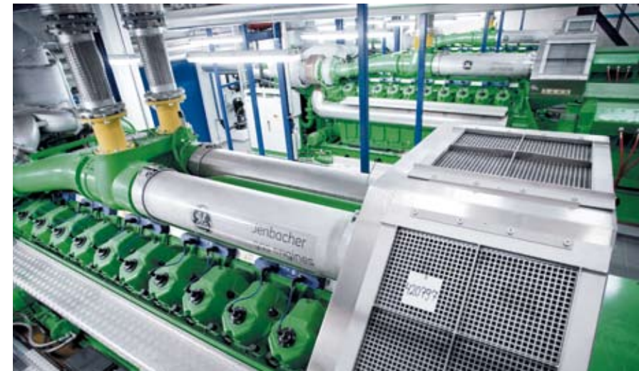
▲ The engine room: three reciprocating engines operate on the biomass-derived fuel from the ANDRITZ Carbona technology.
