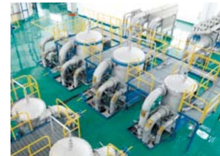
Screens and cleaners in the ANDRITZ stock preparation plant. ▶
