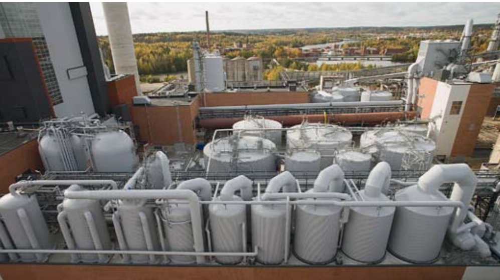
▲ Andritz delivered a seven-effect evaporation plant as part of the project and also the methanol liquefaction plant. Secondary condensates are stripped and collected in four streams – all of which are reused by the mill.
