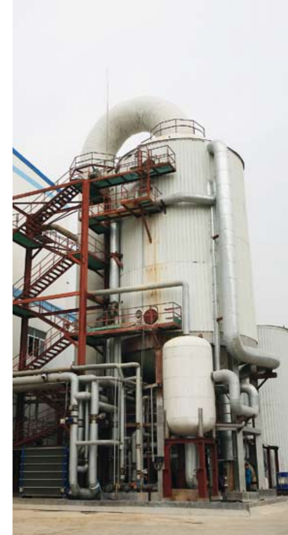
▲ Andritz supplied MVR evaporation technology to process the effluents from the mechanical pulping process and allow their re-use – the first in China to be used in this way for effluent evaporation.
