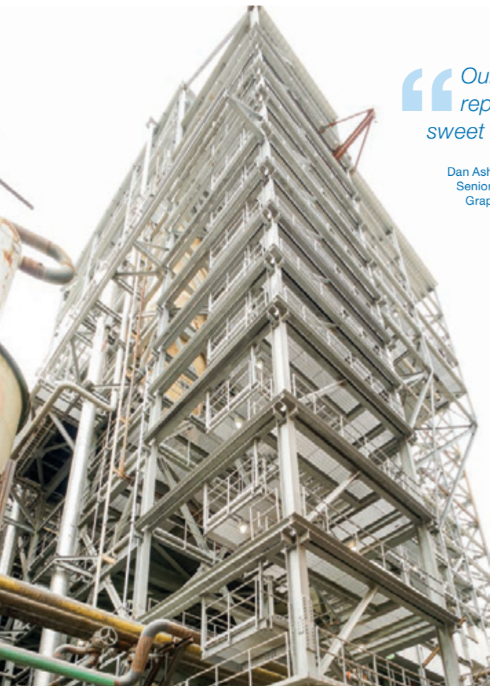
▲ Due to the tight location, the boiler was erected in a unique way. A corner stair support was eliminated so that erectors could bring in the boiler bottom last after other modules were lifted into place.
