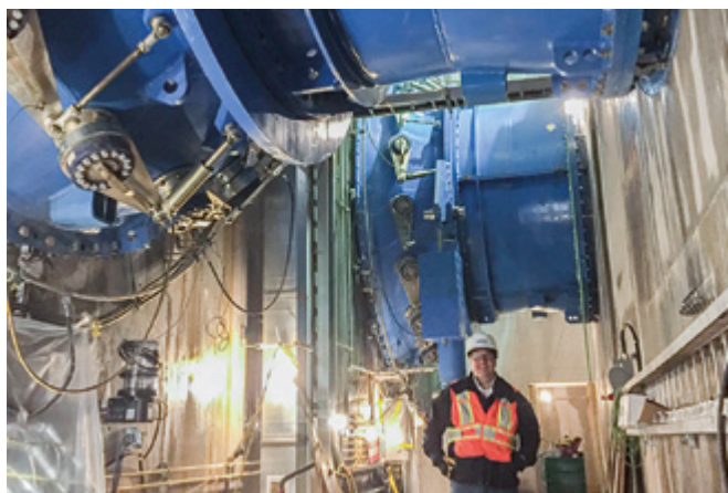
Turbine Bulbe installée
