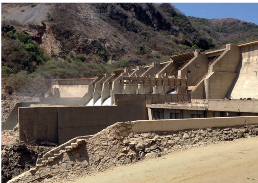
La Venta hydropower plant
